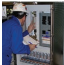
Control and Monitoring
